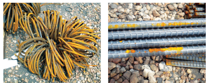
a) Example of rust on small diameter hoops. b) Example of rust on straight bars.
