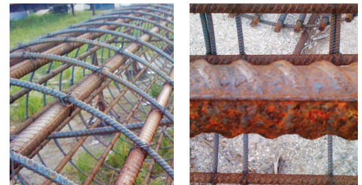
a) Column cage showing general corrosion of the reinforcement. b) Close up view of a longitudinal bar.
