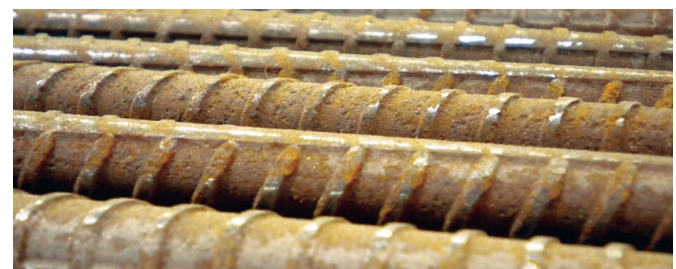
Figure 6 – The tight rust on these bars has not impaired the deformations and would not be detrimental to bond.
